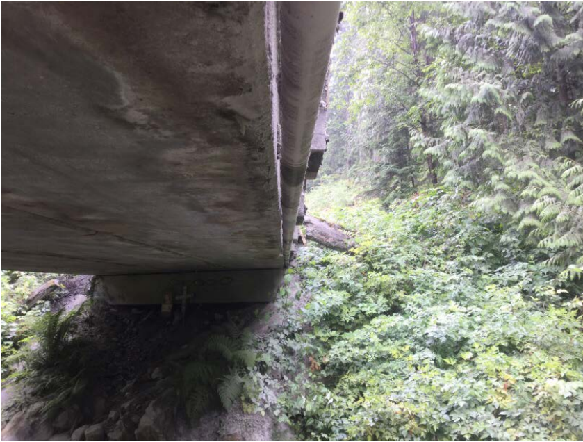
Utilities attached to superstructure
